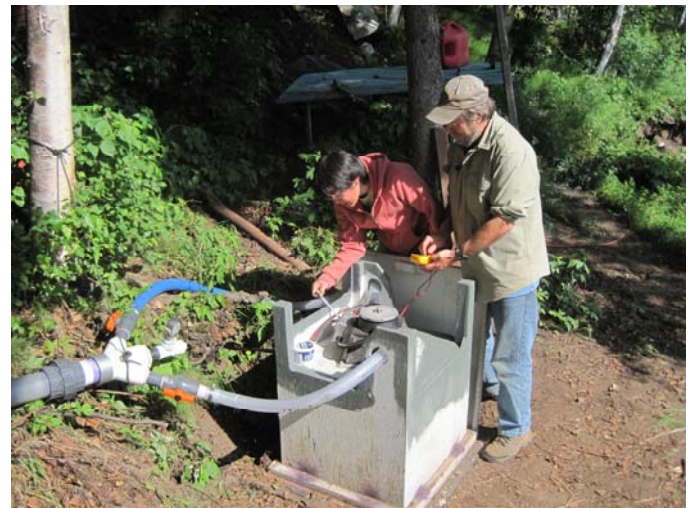
Rapids Research new water power system at main camp, 2010
