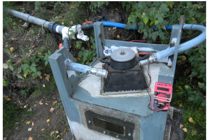
Rapids Research new water power system at main camp.
