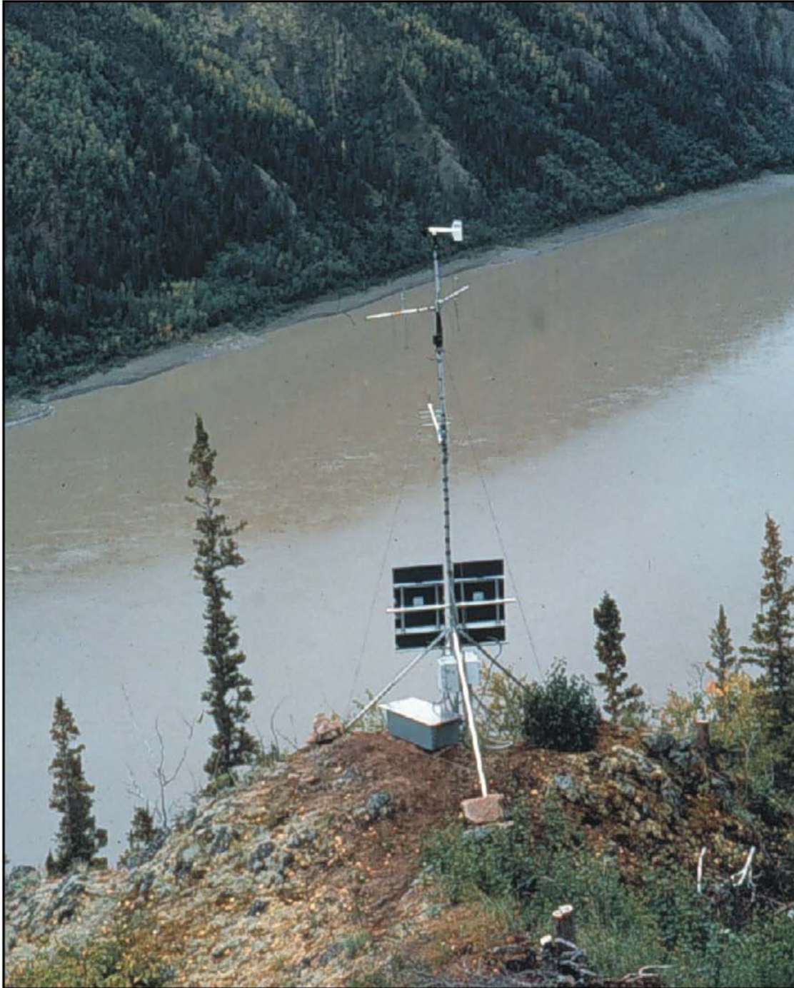
Figure 27. A remote, radio receiving station located high on a bluff along the Yukon River. Solar panels (dark rectangles low on the tower) charge the batteries that power the receiver. Antennas mounted high on the tower point upstream and downstream, allowing the passage direction of radio-tagged fish to be determined based on the strength of the radio signals. In recent years, numerous receiving stations such as this have been deployed around the Yukon and Kuskokwim River drainages to track fish migrations. Photo by J.H. Eiler, NMFS.
