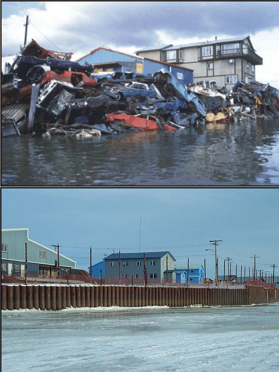
Figure 89. Historical bank stabilization efforts with old cars, waste barrels, and other debris piled over the banks on the Bethel waterfront (top image; photo by J. Barker). Similar situations can be encountered at smaller scales in many rural communities along the Yukon and Kuskokwim River drainages. By contrast, the modern waterfront in Bethel is more effective at preventing erosion and more ecologically sound (bottom image; photo by S.J. Miller, USFWS).
